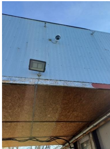
PHOTO 21. PEOPLE COUNTING CAMERA INSTALLED AT HIDEPARK
