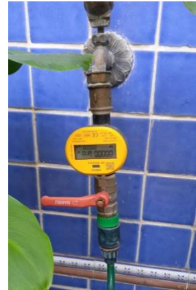
PHOTO 5. FLOW METER INSTALLED AT THE PATIO HYDRANT 22
