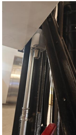
PHOTO 10. INDOOR DEVICE. CO2 SENSOR, 2
