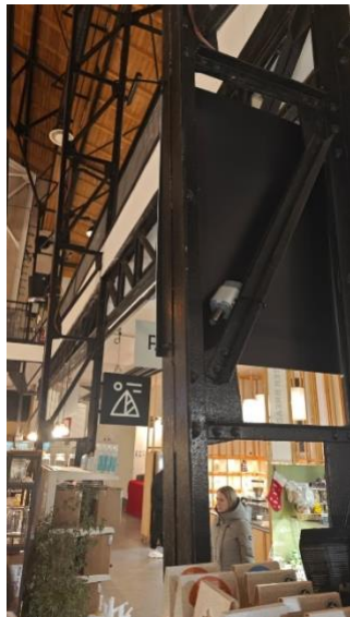
PHOTO 9. INDOOR DEVICE. CO2 SENSOR, 1
